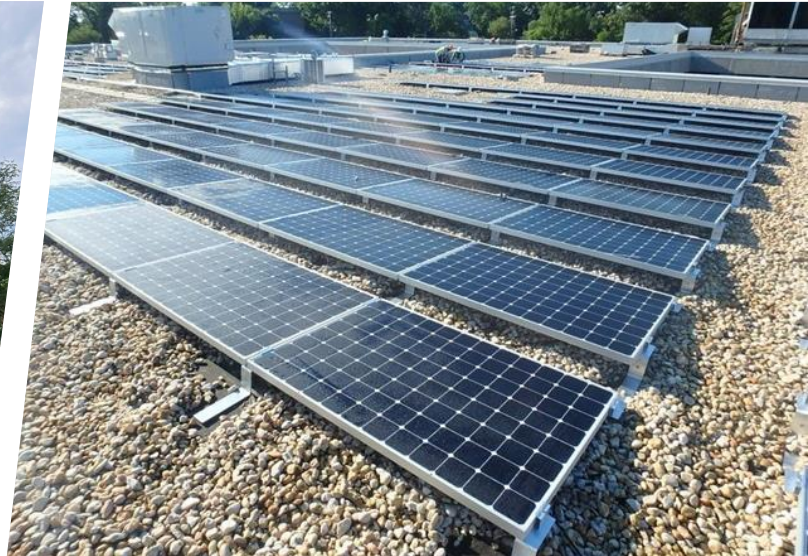
129 newly installed rooftop solar panels
